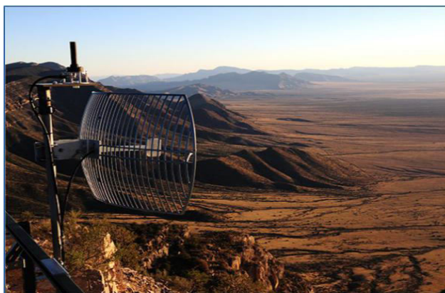
Figure 2: One LocataLite installed on a mountaintop at White Sands Missile Range.
